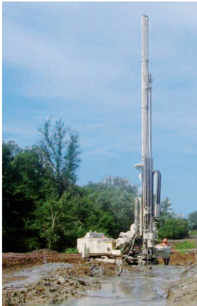
TWS1400-RAPTOR in cantiere, equipaggiata con traliccio jetting L = 12000 mm (lunghezza totale Mast: 18580 mm) TWS1400-RAPTOR on jet-grouting job site, equipped with jetting trestle L = 12000 mm (Mast total length: 18580 mm)
